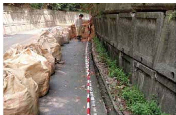
Figure 4 Sand sacks on the road on the first time the landslide occurred (at position 7 in the Figure 7)
