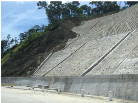
Figure 8 Concrete retaining wall and slope solidification combined with surface drainage for landslide in Da Nang city
