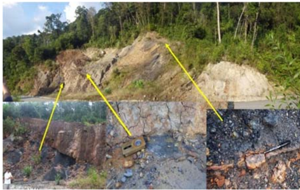
Figure 13 Coal layer, landslide No.21.
