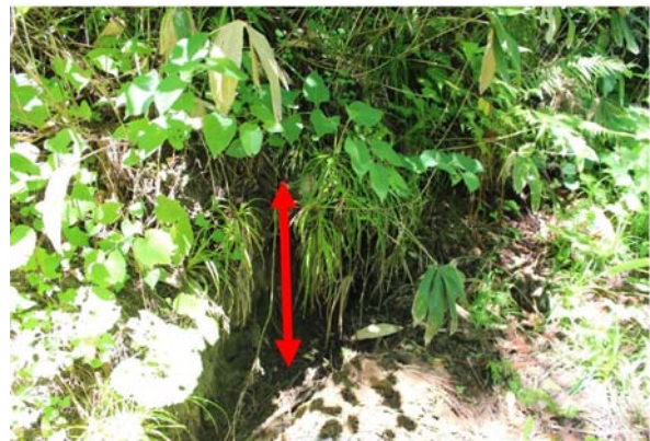
Figure 5 Minor scarp near the toe of slope
