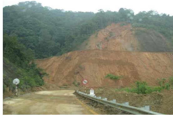
Figure 3 Landslide at Lo Xo Pass on HCM Route
