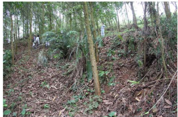
Figure 3 Some distinctive shallow landslide characteristics around KM95 landslide
