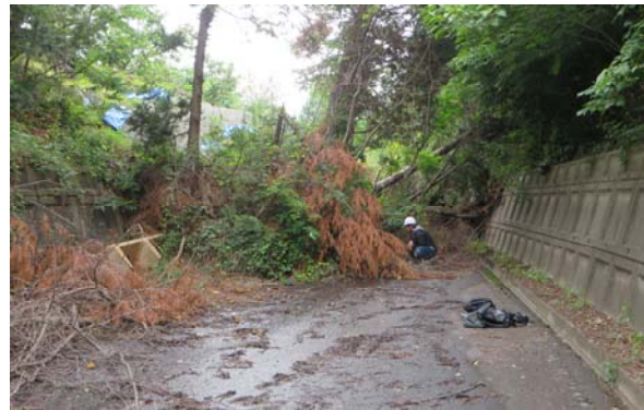
Figure 6 The road on the 2nd time landslide happened (the position 4 in the Figure 7)
