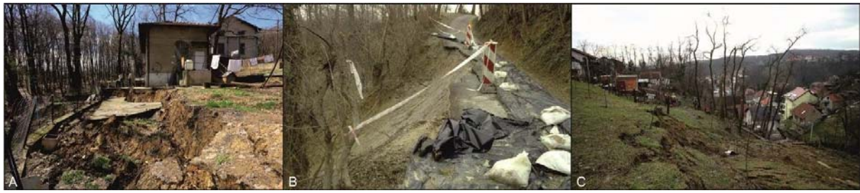
Figure 2 Examples of landslides endangering/damaging houses or public roads in the winter of 2013 in Zagreb (Bernat et al. 2014a).
