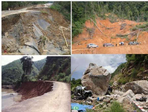
Figure 10: illustrates typical landslides often occur in HCM-Vietnam route
