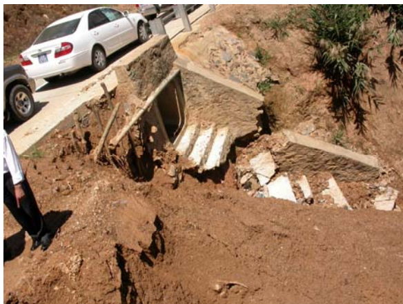
Figure 5 Erosion in Ho Chi Minh route
