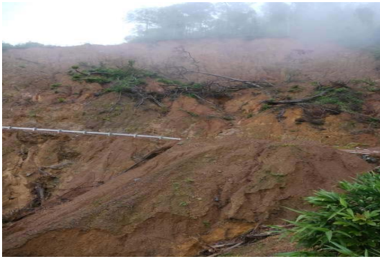
Figure 2 Landslide on HCM Route
