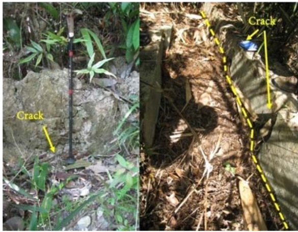
Figure 8 Cracks on top of slope and concrete ditch at landslide No.21.
