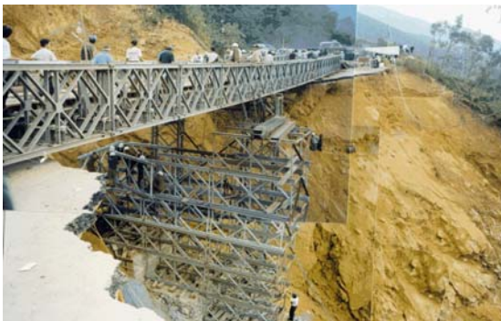
Figure 4 Landslide on Road No.1
