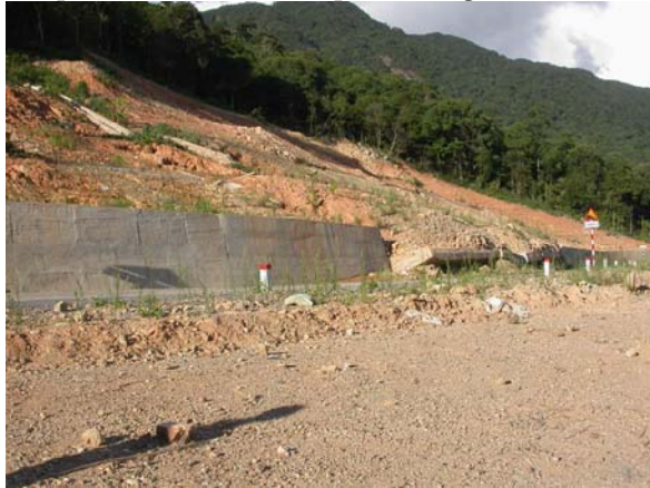
Figure 3 Landslide on Ho Chi Minh route
