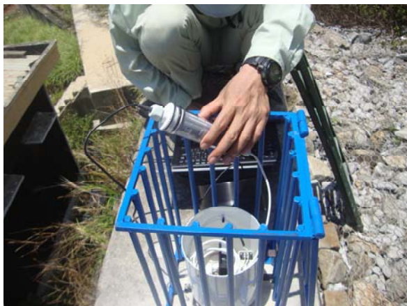
Figure 10 Rain gauge installed in Hai Van station
