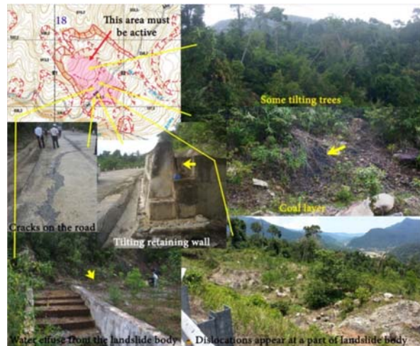
Figure 9 Some evidence of landsliding was observed at a part of landslide No.18.
