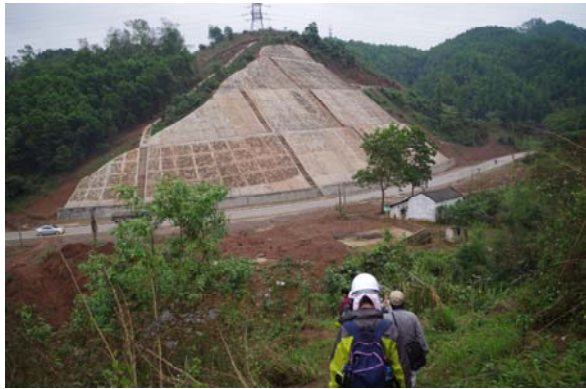
Figure 1 Overview of the KM95 Landslide
