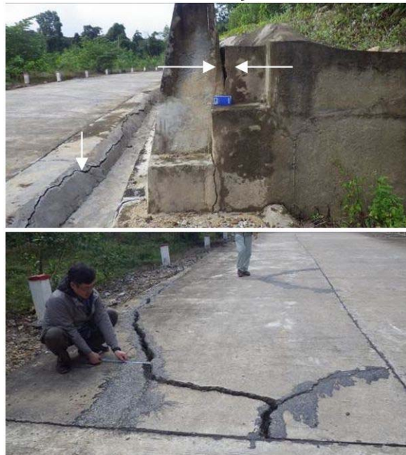
Figure 21 Effects of landslides on a 400-m stretch of the road near No. 356
