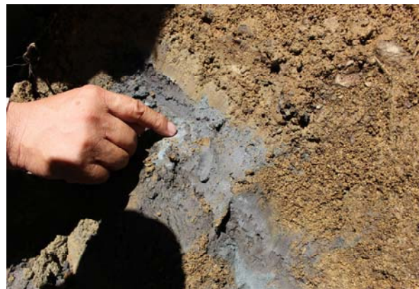
Figure 6 Sliding surface at the toe of landslide area
