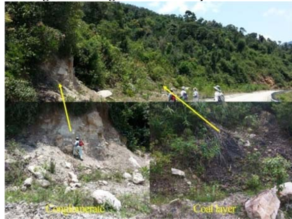
Figure 11 Coal layer and fractured rock consisting of sandstone, mudstone and conglomerate on landslide No.18.
