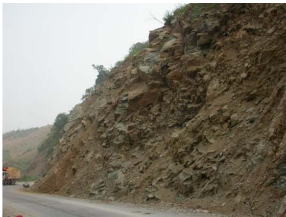
Figure 9 Rock fall on national road No.37
