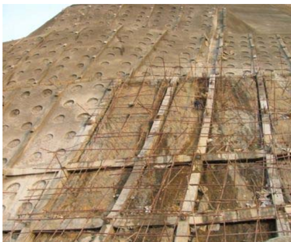
Fig.9 Combination of reinforced concrete frames and OVM anchors to prevent landslide on Da Deo Pass
