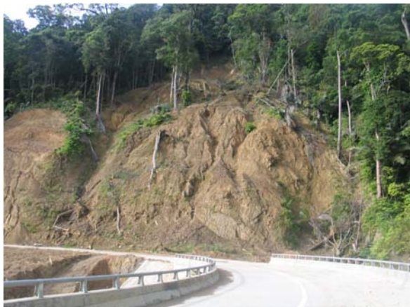
Figure. 9 Landslide at section 3
