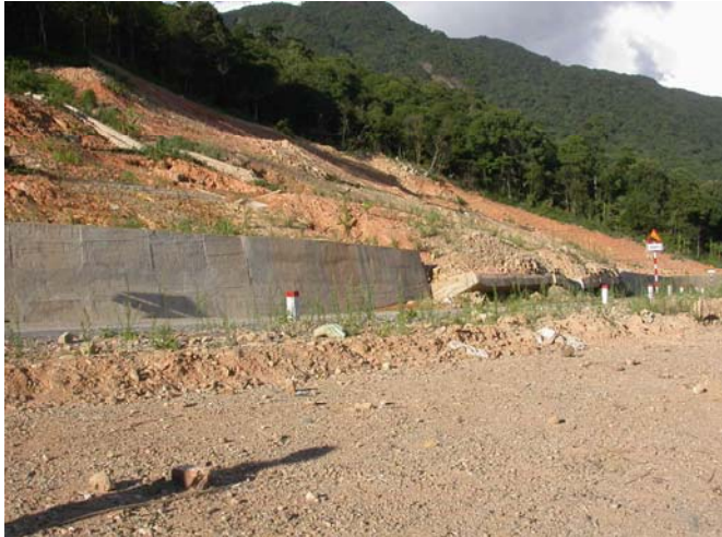
Figure 3 Landslide on Ho Chi Minh route
