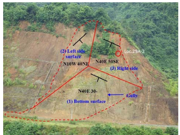
Fig. 13. Landslide No.029 on HCM route
