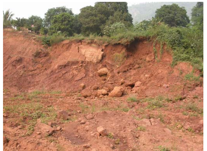
Figure 7 The topple in national road No.6
