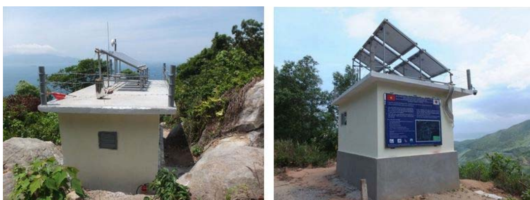
Fig. 5. Monitoring hut (BHH) in landslide slope and monitoring station (TSH) in opposite stable slope (Asano et.al 2016)
