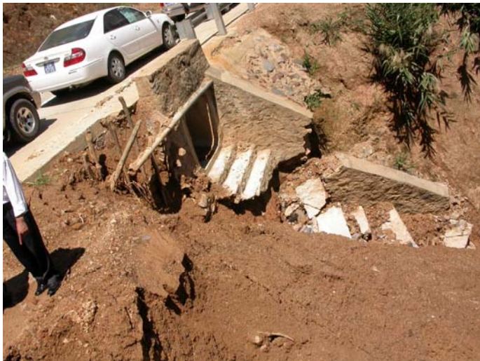
Figure 5 Erosion in Ho Chi Minh route.
