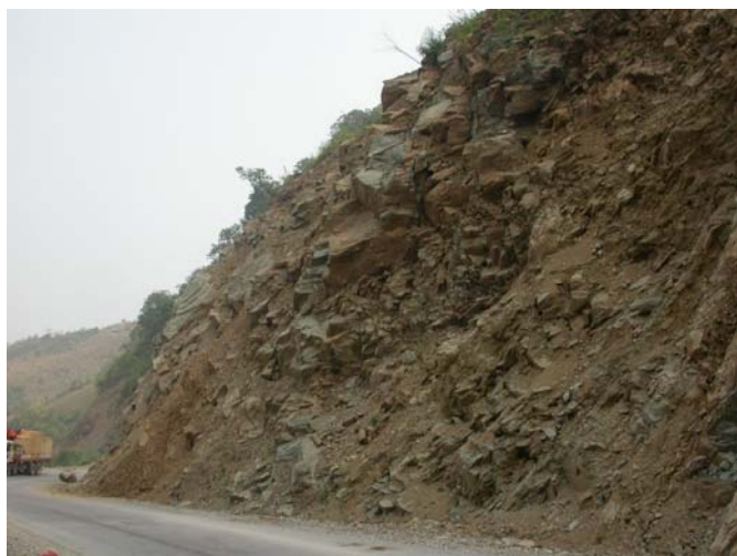
Figure 9 Rock fall on national road No.37
