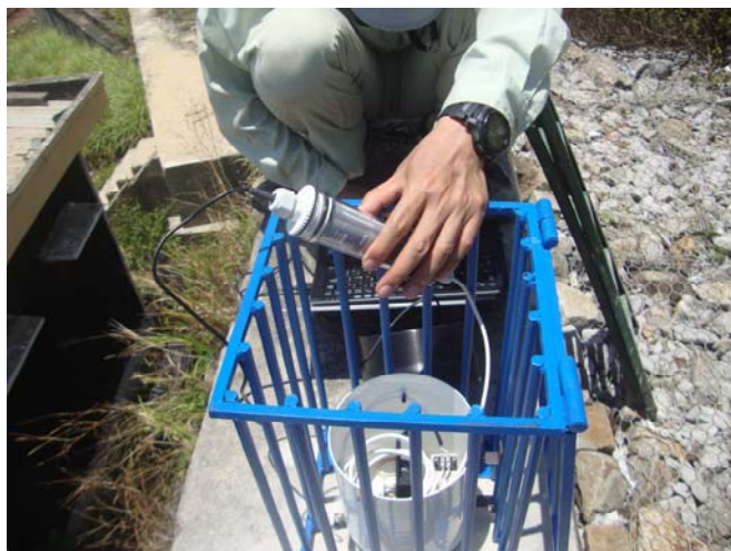
Figure 10 Rain gauge installed in Hai Van station
