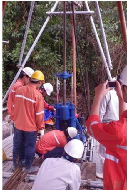
To pay attention on the installation work for safety, preliminary observation of rain and displacement was conducted.
