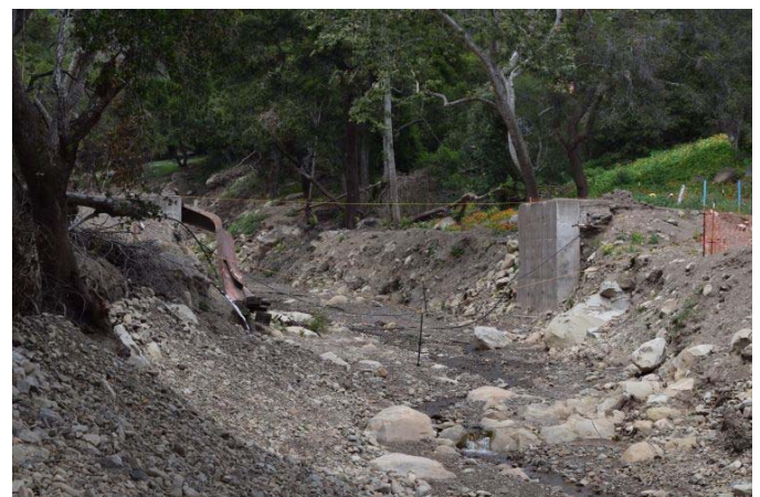
Figure 1 A bridge washed away due to waterway blockade.
