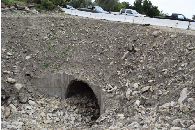
Figure 8 Depth of debris mass that came down and blocked the culvert as well as the elevated roads.
