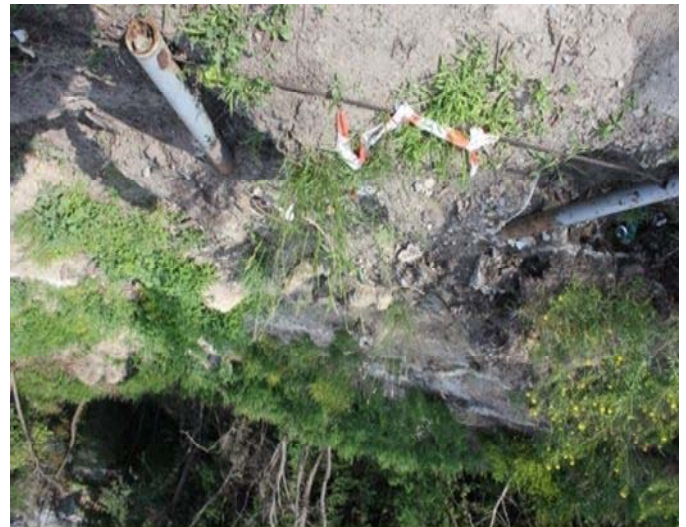
Figure 6 An example of the active development of landslide processes with active developments and erosion processes on the slope of the Church.
