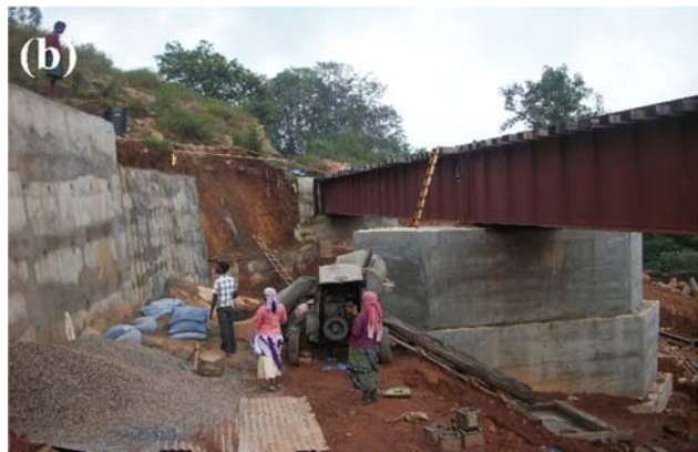
Figure 7 Aravankadu 2009 landslide (a) View of landslide (b) Retaining wall near new railway bridge
