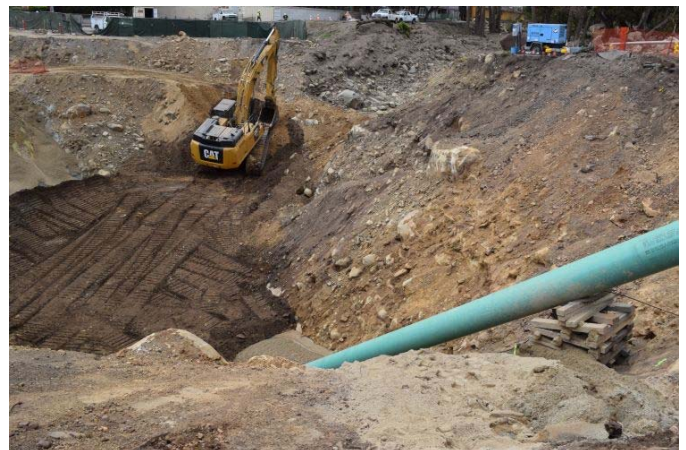
Figure 7 Gas pipeline that were damaged during the debris flow event and caught fire.
