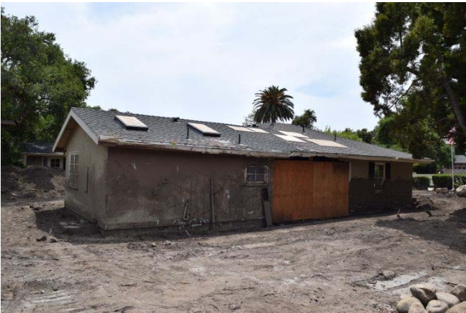
Figure 3 Damage to buildings due to diversion of debris mass towards residential area.
