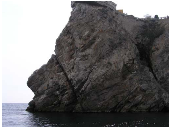
Figure 2 – The northern view. The huge crack separating some part of the rock from the main cliff part and a range of smaller cracks covering the whole Swallow's Nest castle base could be seen on the figure 2.
