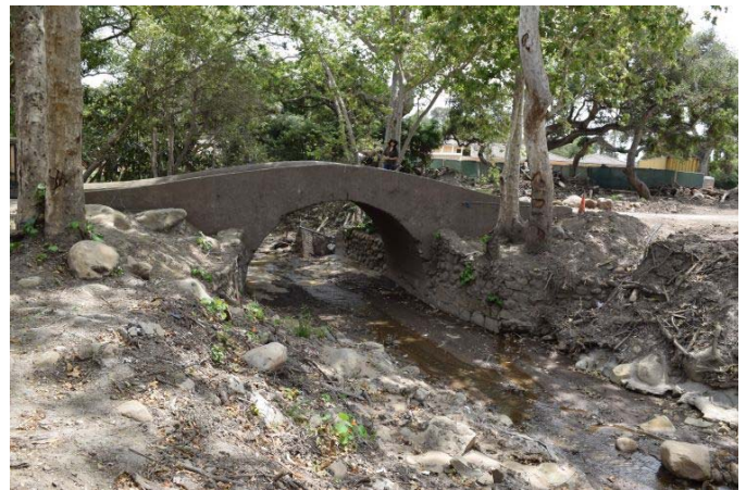
Figure 6 Culvert structure, right bank of which had debris flow diversion that caused a massive loss of properties.
