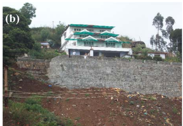
Figure 5 Retaining wall at Chinnabikatty (a) Top view from road (b) Over all view from toe
